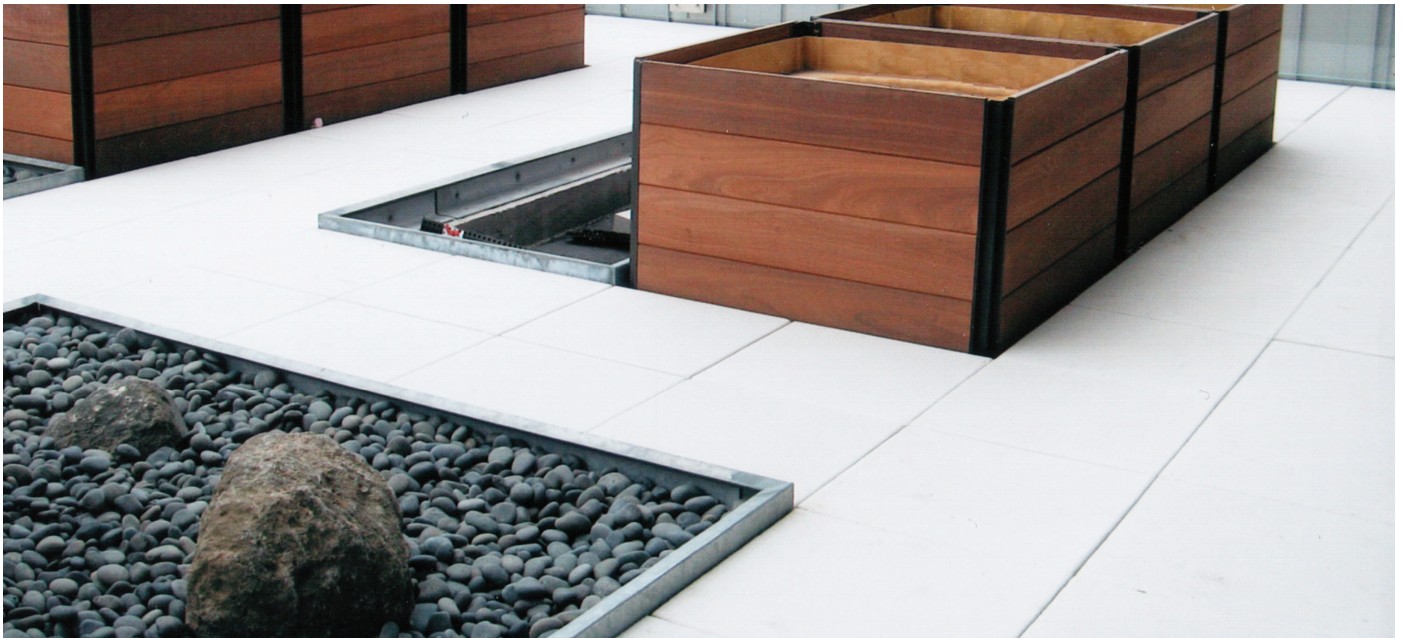
TORONTO, ON - SOLAR REFLECTIVE ROOF BALLAST SLABS
